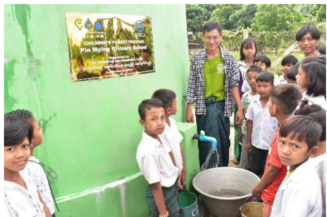
Rainwater tank installed at a school (Myanmar)
